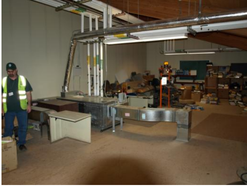
Fleet HVAC AHN #2
