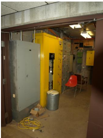
Fleet electrical room – motor control cabinet
