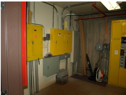
Operations electrical panels
