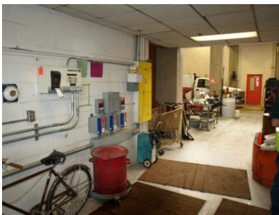
Fleet light duty electrical panels
