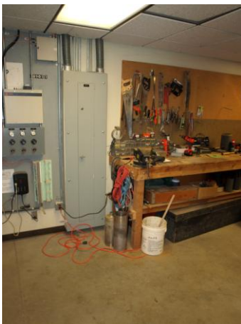
Operations Lab electrical panel
