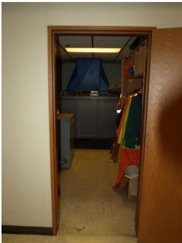
Operations Sign Shop booster fan
