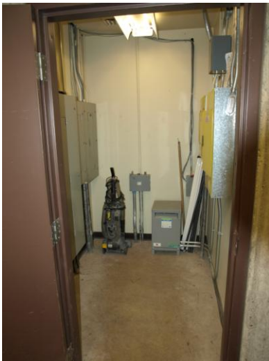
Administration 1 st floor electrical closet
