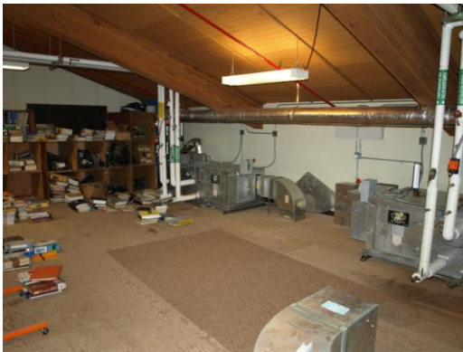
Fleet HVAC AHN #3
