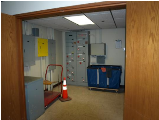
Operations motor control cabinet electrical panels
