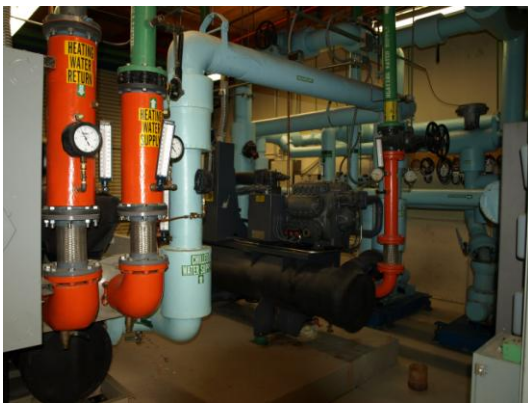
Operations mechanical room chillers #1 & #2
