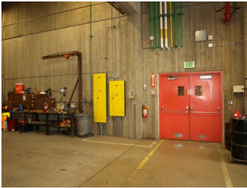
Fleet heavy duty electrical panels
