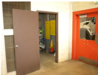
Fleet heavy duty electrical closet
