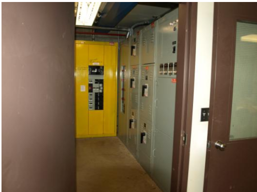
Operations electrical distribution
