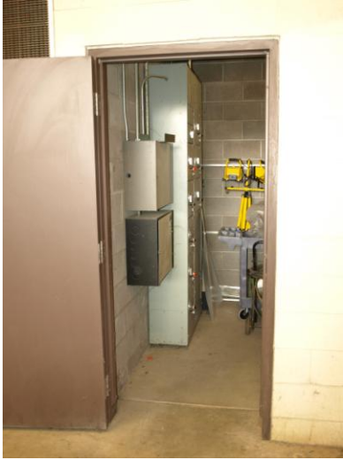
Fleet heavy duty electrical closet
