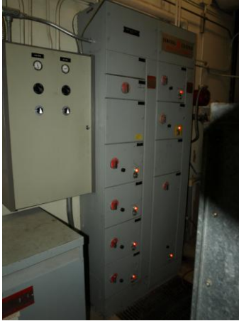
Administration mechanical room (M.C.C)
