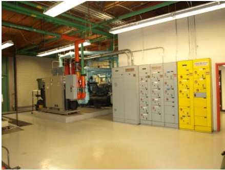
Operations motor control cabinet
