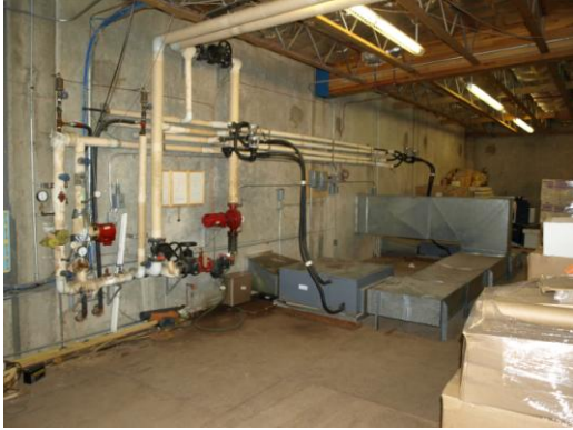
Warehouse HVAC (office unit)
