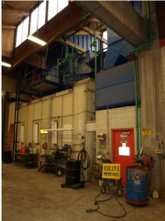
Fleet heavy duty HVAC
