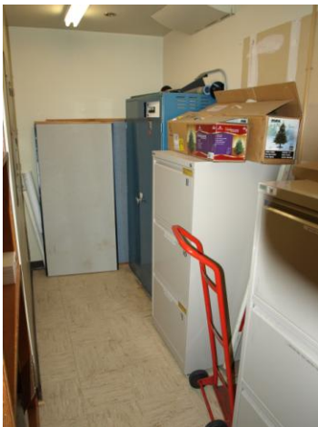
Administration 2 nd floor electrical closet
