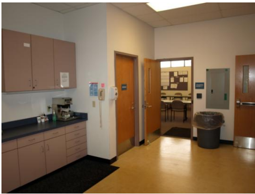
Operations training rooms electrical panel
