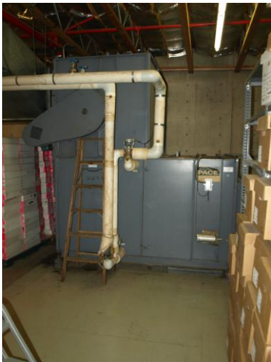
Warehouse HVAC main unit
