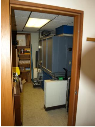
Operations booster fan (mechanical room)
