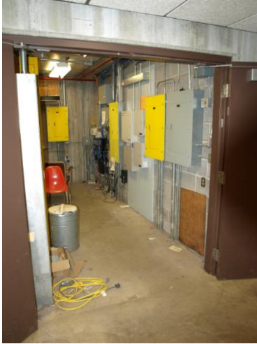
Fleet electrical room – motor control cabinet
