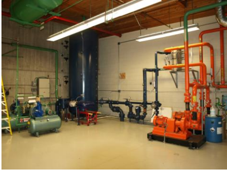
Operations mechanical room
