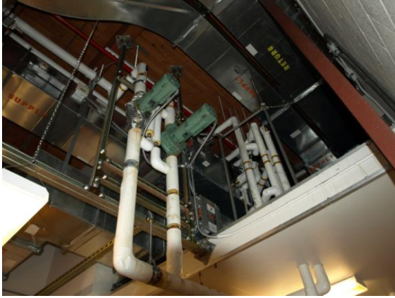
Operations training rooms HVAC (AHN 1-4)
