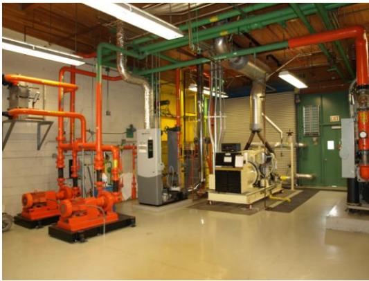
Operations mechanical room (E.D.G)
