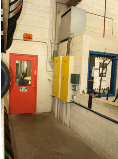
Fleet tire shop electrical panels
