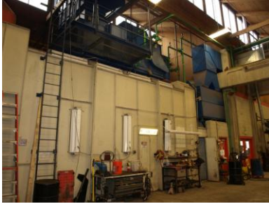
Fleet heavy duty HVAC
