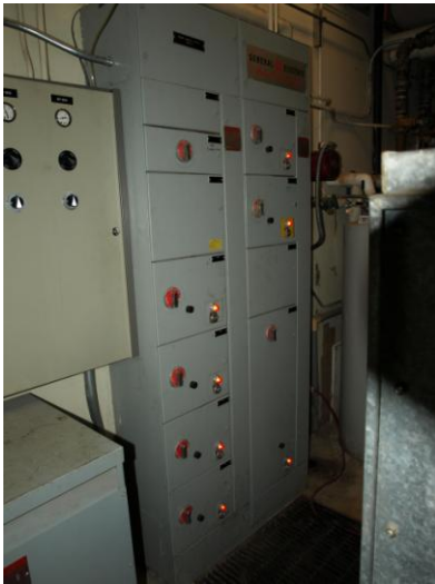
Administration mechanical room (M.C.C.)
