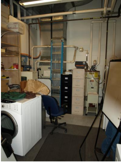
Building H HVAC indoor unit
