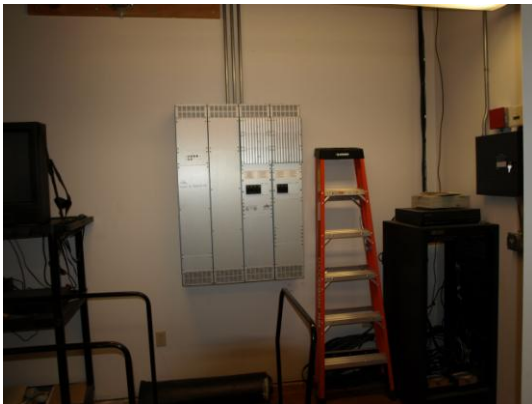
Operations lighting control (mechanical room)
