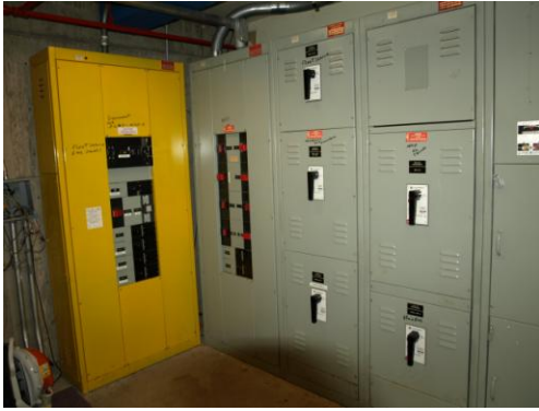
Operations main panel
