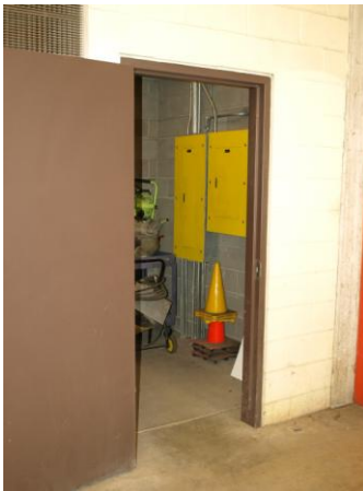
Fleet heavy duty electrical closet
