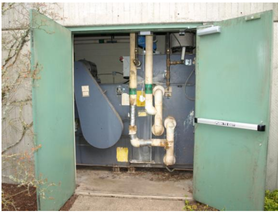
Operations HVAC mechanical room main unit
