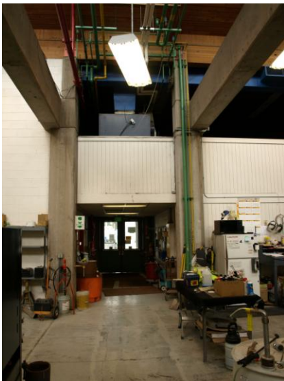
Fleet light duty HVAC – heating only
