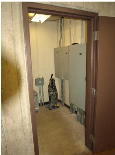
Administration 1 st floor electrical closet
