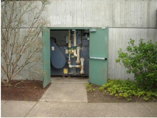
Operations HVAC mechanical room
