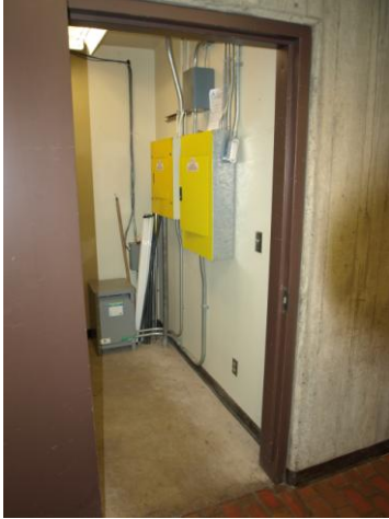
Administration 1 st floor electrical closet
